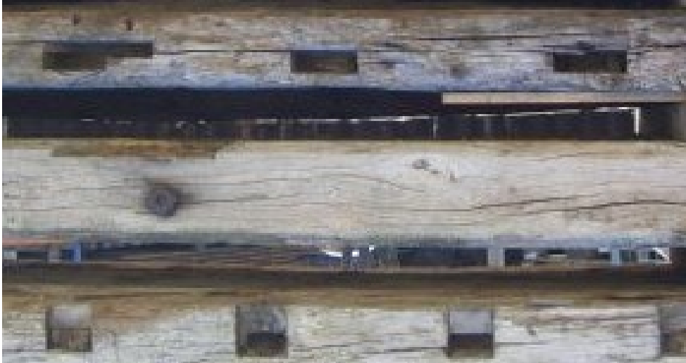
Empty mortise joints
